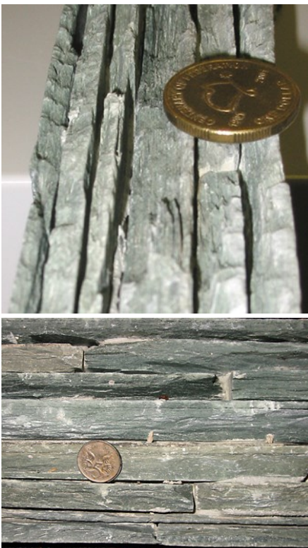
Figure 1. The attached photo is an example of an unstable stacked cladding stone, made by gluing together laths of Micaceous Schist. As can be seen some of the laminations are breaking along the cleavages. The epoxy adhesive was applied onto the cleavage which then breaks parallel to it.
